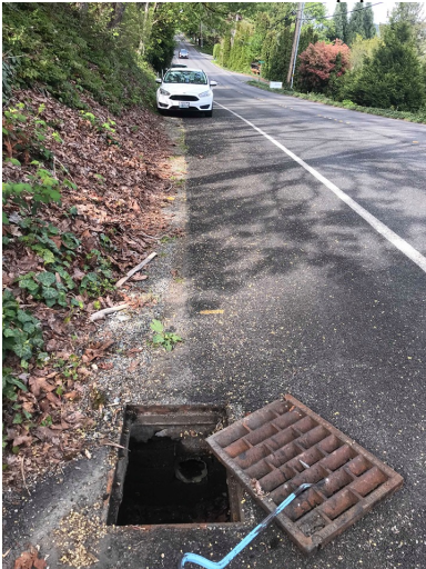
Photo 8 (Looking N): Type 2 Manhole (#3). Inlets from the West, South, and East side of MH.
