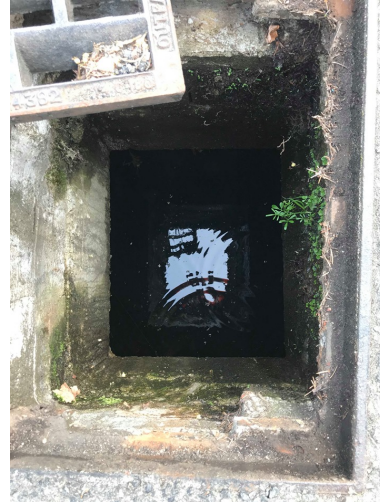
Photo 4 (looking into CB #2): Type 2 CB (#2). Two inlets from south and east side. Outlet flowing north.
