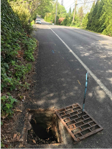
Photo 1 (looking N): Type 1 CB (#1). Not shown in Mercer Island GIS. All drainage on site will be routed to a new proposed catch basin in the ROW which will outlet to CB (#1).
