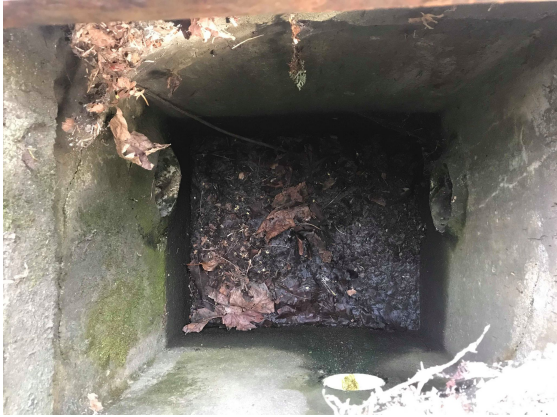
Photo 2 (looking into CB #1): Type 1 CB (#1). Two inlets from south and east side. Outlet flowing north.
